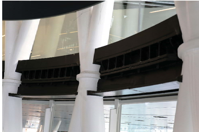
Fig. 11 Plate N° 2, Between 3rd and 4th Floors. Photograph taken from inside tube N° 5. (Copyright: sendai mediatheque)
