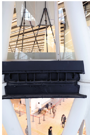
Fig. 12 Plate No. 1, Between 1st and 2nd Floors. Open Square can be seen on the 1st-floor level. (Copyright: sendai mediatheque)
