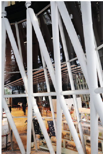
Fig. 5 View from Interior of Tube N° 5 at 1st Floor. The Open Square can be seen through the glass of the tube. (Copyright: sendai mediatheque)
