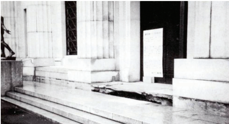
Fig. 4 The building tilted westward at a 5-degree angle, The Kobe City Museum (Copyright: The Kobe City Museum from “Report of Investigation for Museums in the Great Hanshin-Awaji Earthquake I / II”)
